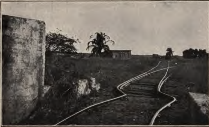
A. Subsidence of the ground with consequent tilting of buildings in the Victoria Battery, Port Royal. The kink in the railway track is over a fault.
